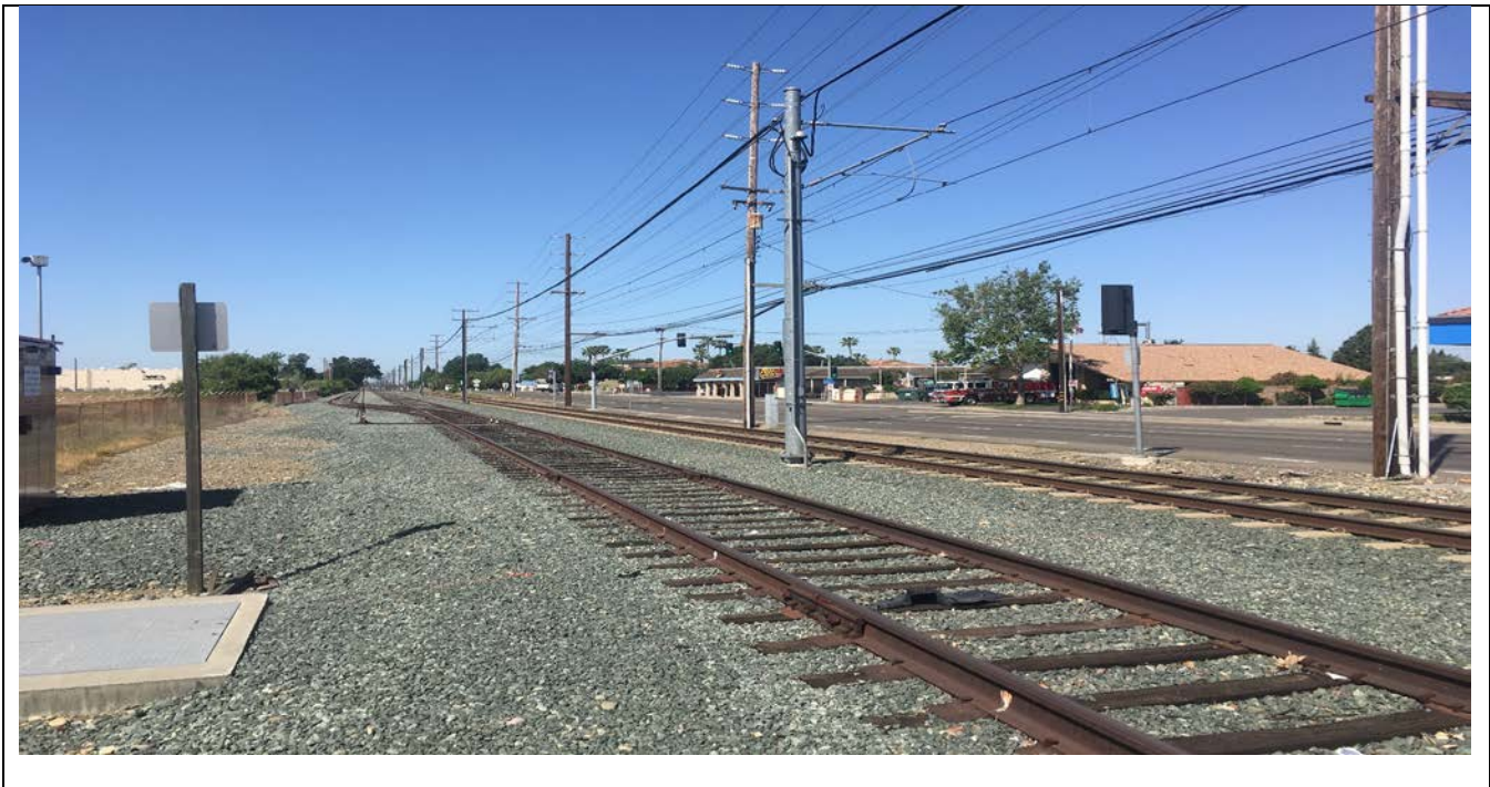
Viewpoint 7. Looking south at Folsom Boulevard from Nimbus Road. The light rail tracks, OCS, chain-link fencing around the Aerojet property, a portion of SacRT wayside equipment, wood power poles and overhead electrical lines, Folsom Boulevard and associated traffic signals, commercial development, and scattered trees are visible in the foreground, middleground, and background.
